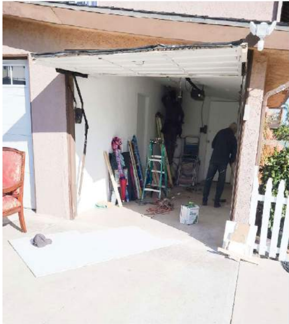
Single Car Garage before new outlets
