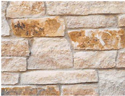
MODERN BUILDING SUPPLY, ' RATTLESNAKE LIMESTONE', OVERGROUT JOINTS
