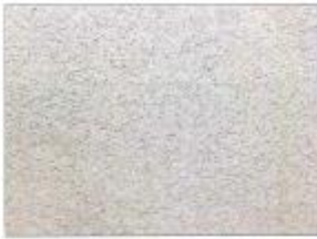
(N) 7/8" SMOOTH COAT STUCCO OVER METAL LATH w/ 2-LAYER GRADE-D PAPER O/ALL WOOD BASE SHEATHING. STUCCO COLOR & TEXTURE COLOR: BEHR W-F-400 SWAN WING
