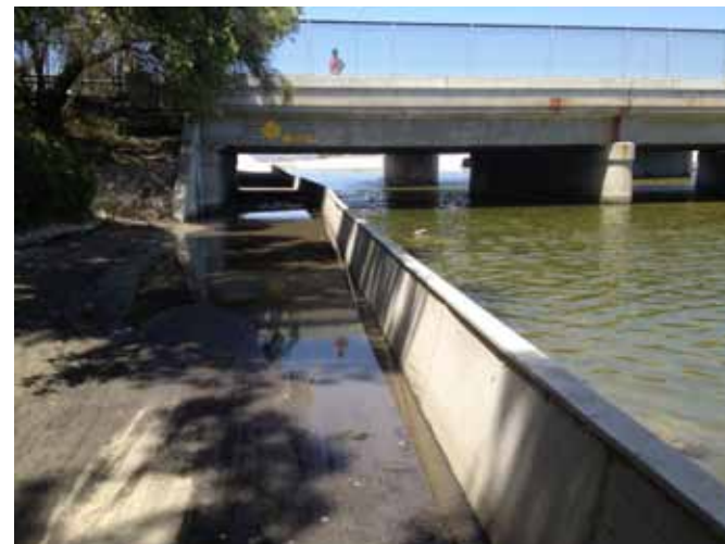
San Juan Creek Trail under PCH Connector/Park Lantern during high tide event (7 June 2012)
