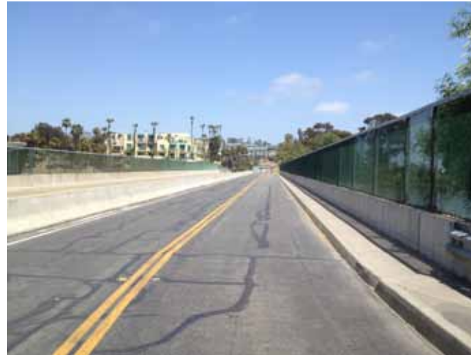
Park Lantern/PCH Connector bridge over San Juan Creek looking southeast toward DoubleTree Hotel
